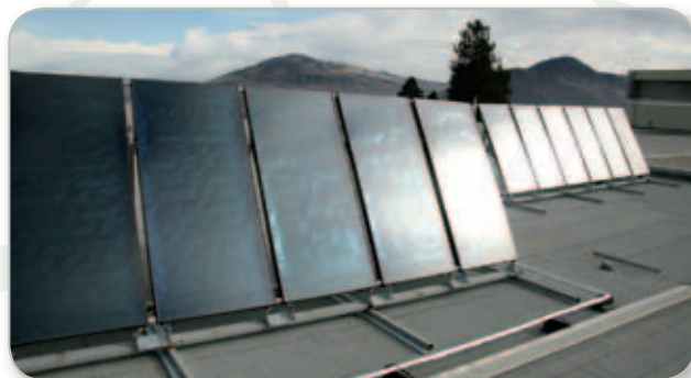
Solar panels on Old Main, the Campus Activity Centre, and Culinary Arts provide hot water heating year-round, reducing energy costs in these water-dependent facilities.
