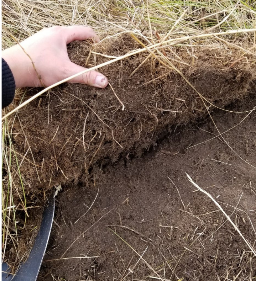
Figure 3.1. The vegetation was peeled back and removed. Soil was salvaged from the root mass and removed evenly from the surface.
