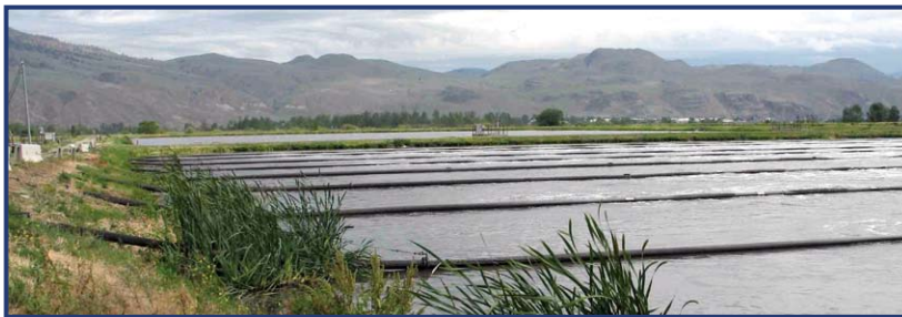
Figure 56. Bubblers within the secondary treatment lagoon mix oxygen into the wastewater. This oxygen is essential to sustain bacteria that feed on and digest the organic matter, converting organic compounds to non-harmful products. Abundant green algae on the surface and shoreline plants reflect the nutrient-rich nature of the waste water. (Photo by R..Turner)
