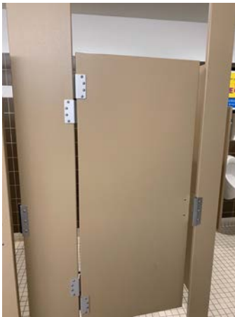
Photo 6.2-1 Stall Door with Gap in Student Union Building
