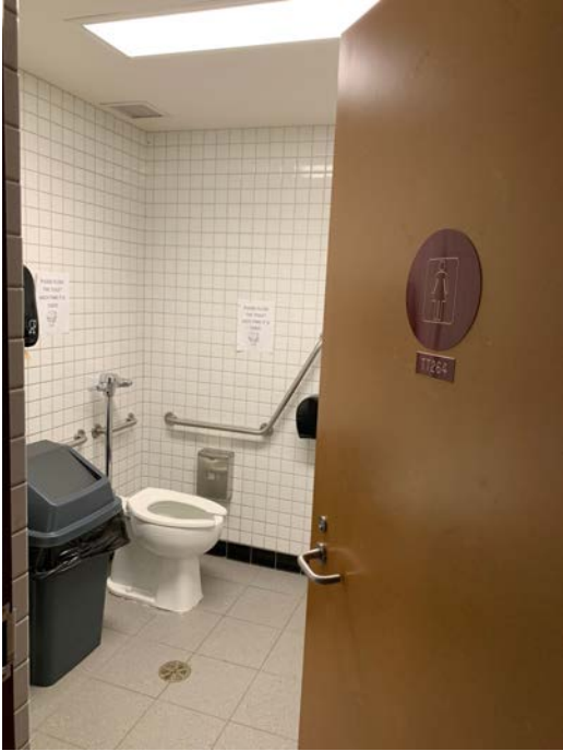
Photo 6.4-3 Signage for Single- Occupancy Washroom in Trade + Tech
