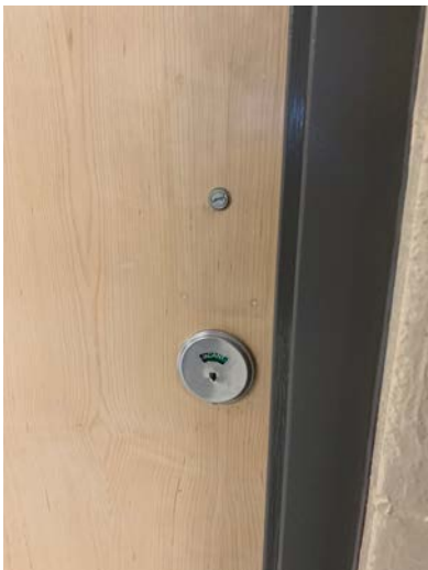
Photo 6.2-3 Lock with Occupancy Indicator in Main Building
