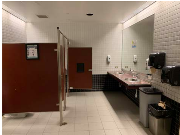
Photo 6.2-2 Stall Doors with Gap in Front of Mirror in Trade and Tech
