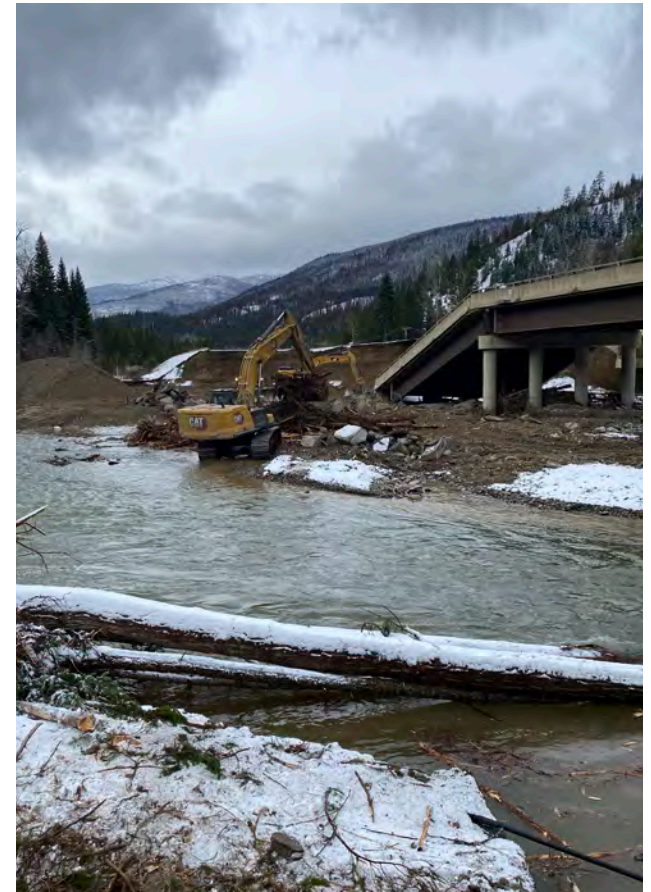
Above: Flooding in fall 2021 caused catastrophic damage to major highways and supply chain networks across British Columbia.
