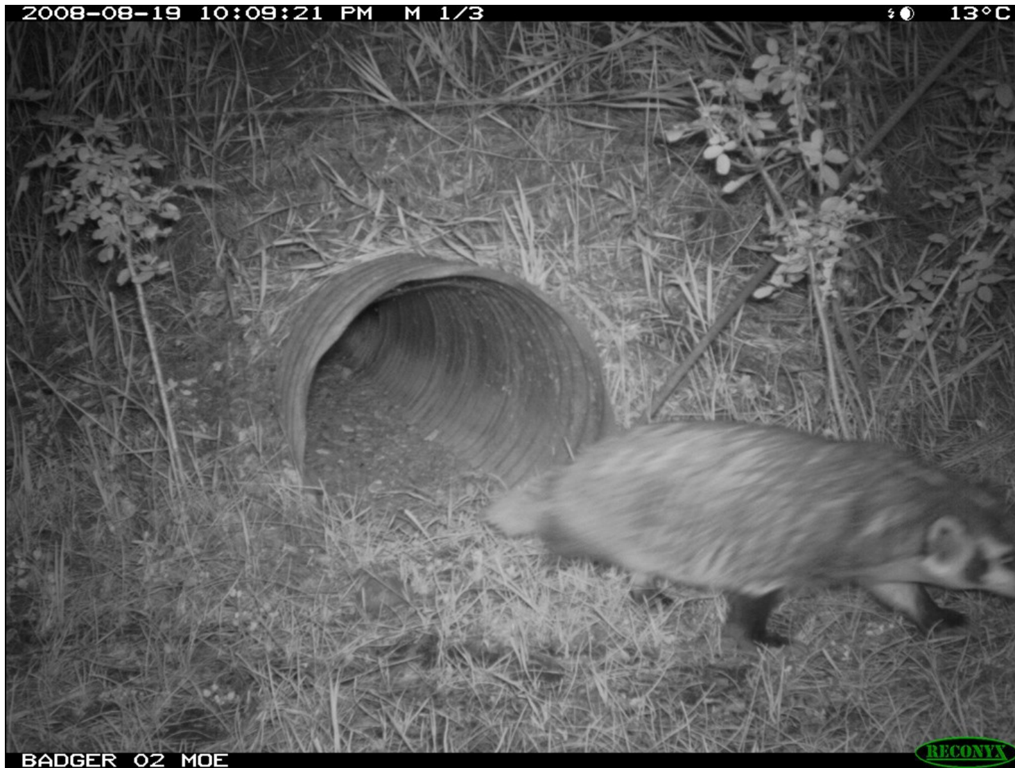
Figure 3.2. Suitable existing underpass structure (500 mm corrugated pipe) with earth substrate bottom used by badgers to pass under Highway 97 north of 100 Mile House BC, Canada, 19 August 2008.
